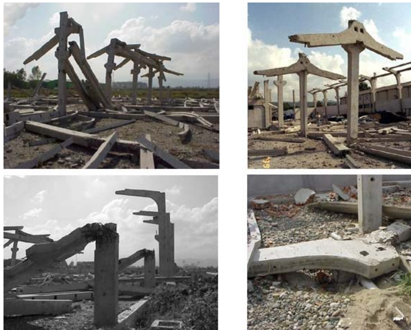
Fig. 7 Colapsul unei hale in curs de executie
