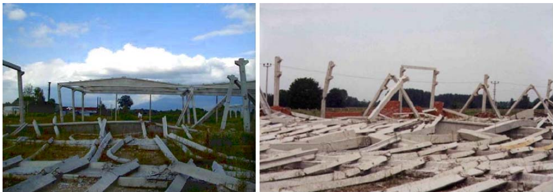
Fig. 2 Colapsul unei hale in curs de executie
